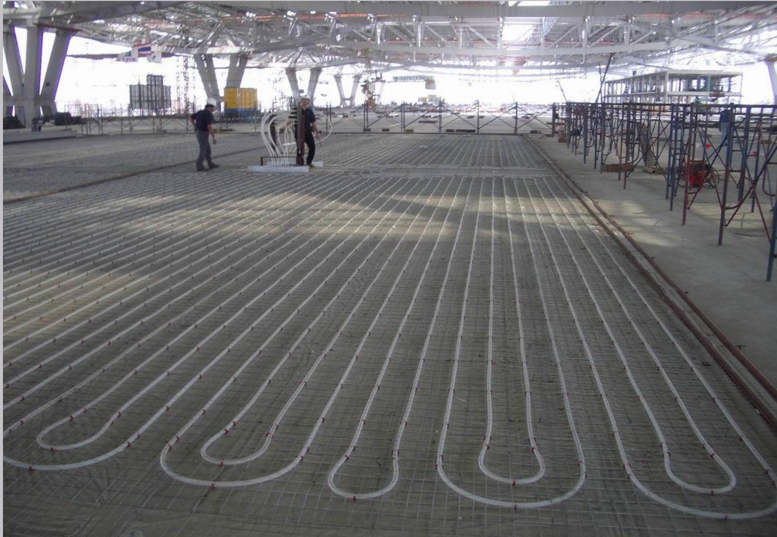
Floor cooling as a heat sink - Bangkok International Airport, Murphy/Jahn Architects
